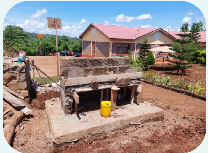
The school water system is powered by solar energy, meaning the children will have abundant water regardless of access to electricity.
