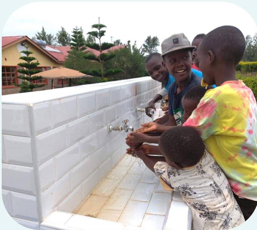
Some of the children at the school excitedly test out the new tap stand!
